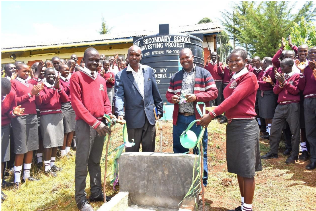
Photo showing Rain water Harvesting System Installed and being handed over at Kaputi Secondary School
