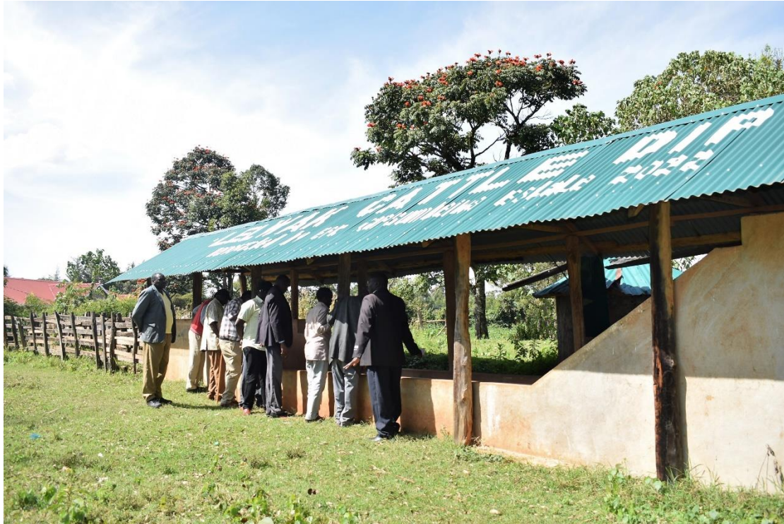
Photo Showing farmers looking on at the crack repairs done inside the dip
