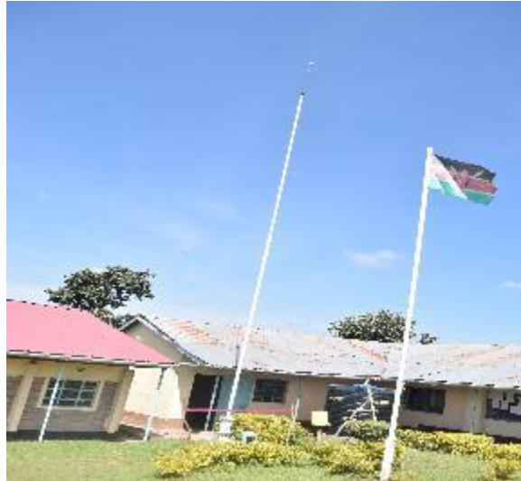
Photo showing lightning arrestor installed at Chepsire Vocational Training Centre
