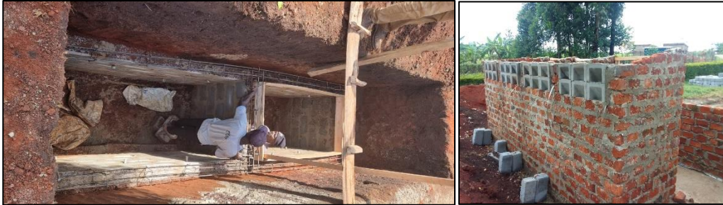
Photos showing progress of the construction of a 4 door sanitation facility at Mosombor Dispensary
