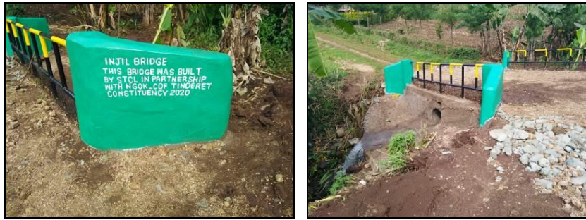
Photos showing one of the complete bridges done by Siret Tea Company with support from the National Government – Constituency Development Fund
