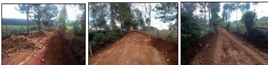
Photos showing Work in progress at Cheptabach Road; in June, 2019, now complete
