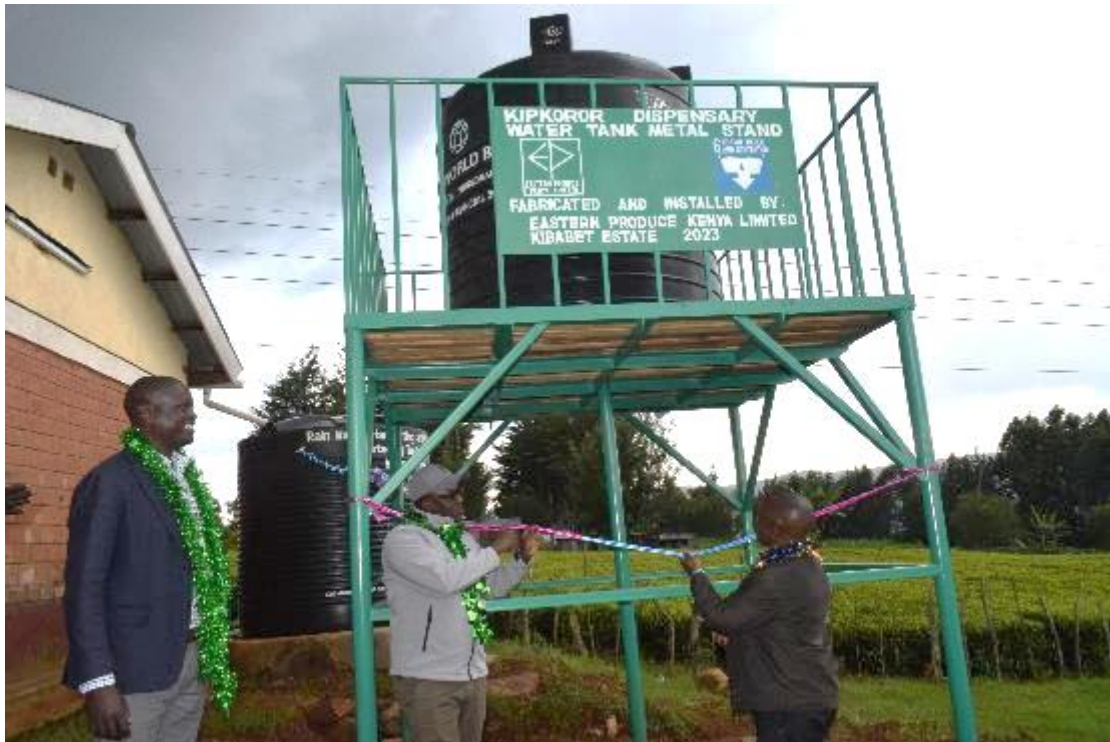
Photo showing Installed water tower at Kipkoror dispensary.
