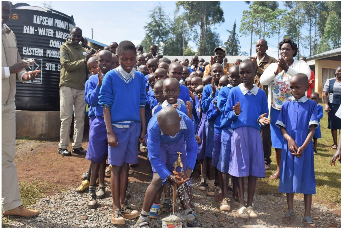
Photo showing Rain water Harvesting System Installed and handed over at Kapsean primary school
