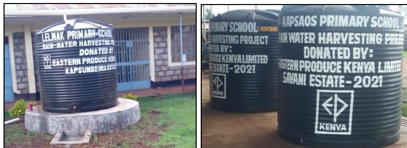
Photo showing a set up Rain Water Harvesting Kit at Lelwak Primary school and branded tanks ready for installation at Kapsaos Primary school
