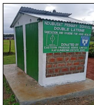
Photo showing a complete double door latrine ready for handing over at Ndbusat primary school
